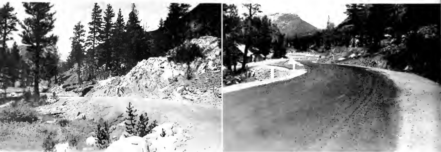
Section of new Tioga Pass Highway looking easterly toward Camp Tioga. Left—Before and (right) after improvement
